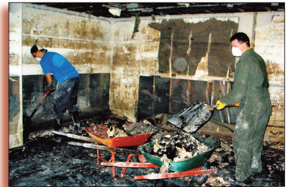
Friends helping us gut out the basement — river muck & sewage — Yuck!!!
