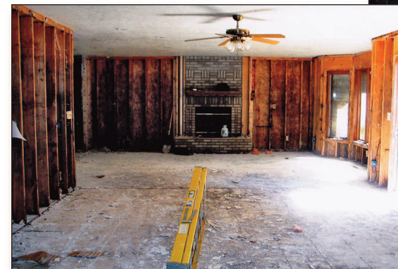
Main Floor — living room — 7 ft. water.
